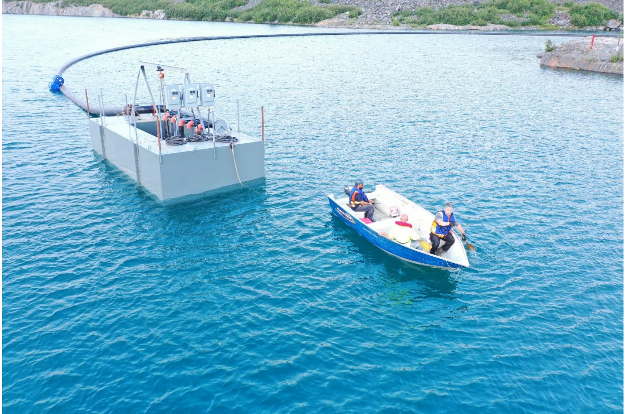
Image 1: Troilus employees position a barge with 3 x 140Hp pumps in the J4 Pit. Water pumped from J4 travels through a pipe for treatment before being released into the surrounding environment.
