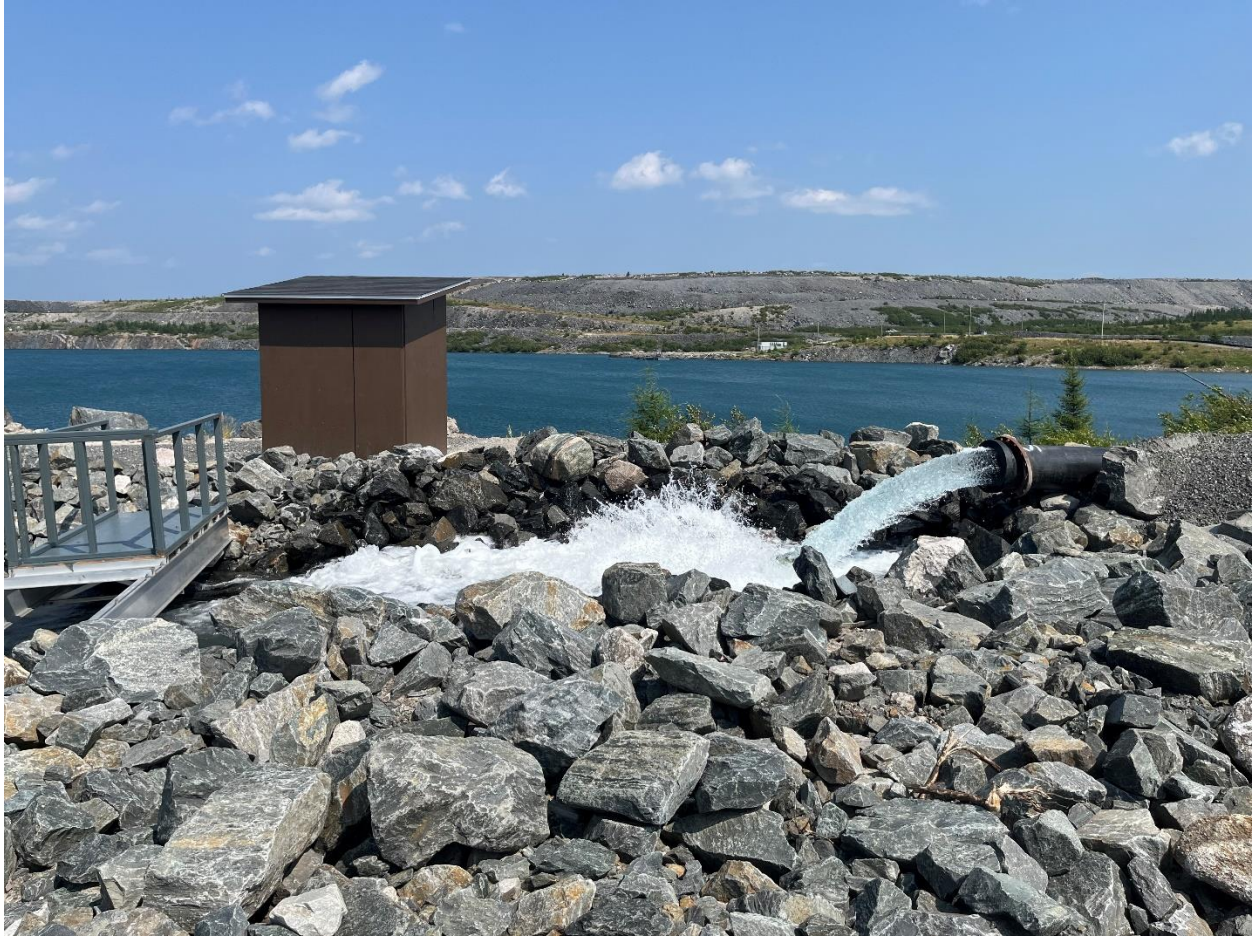
Image 2: Water pumped from the J4 Pit is treated before being released into the environment. Temperature, pH level and flow rate are continuously monitored.
